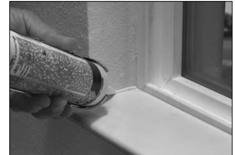
11 Finish off the installation by applying a bead of caulk between the sill and the drywall. Smooth the caulk with a wet finger.
